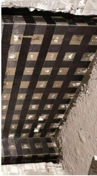
Figure 22 – Example image of a concrete shear wall strengthened through the introduction of carbon fibre reinforcing in both vertical and horizontal directions.
