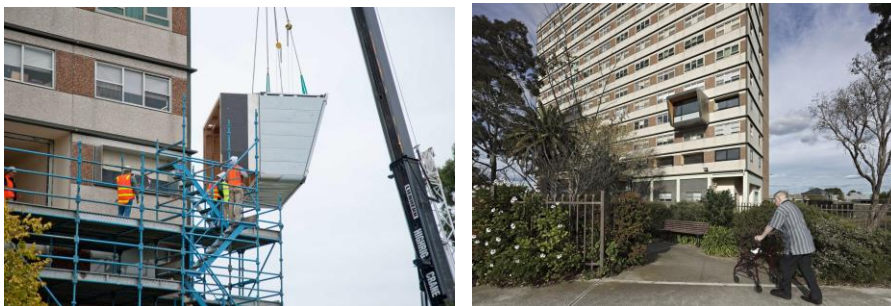
BKK's prefabricated pod being installed onto the existing high-rise building. Photo by BKK.
